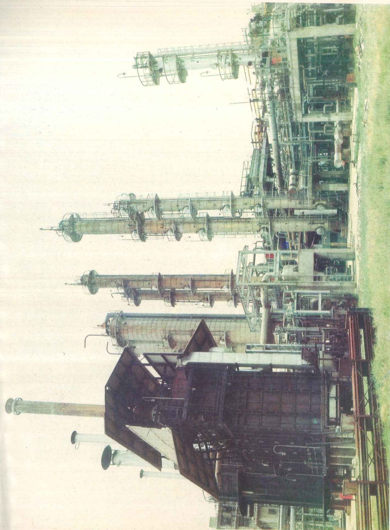
1. Xylene isomerization plant of IPCL, Vadodara, Capacity 50,000 TPA
