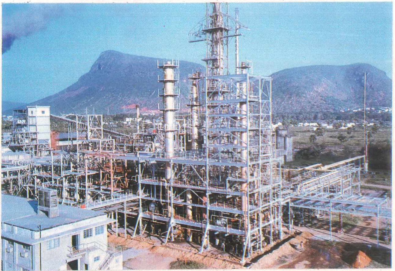
Ethyl benzene Plant at Vizag (Hindustan Polymers Limited)
