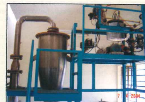
Steam Explosion Digester
