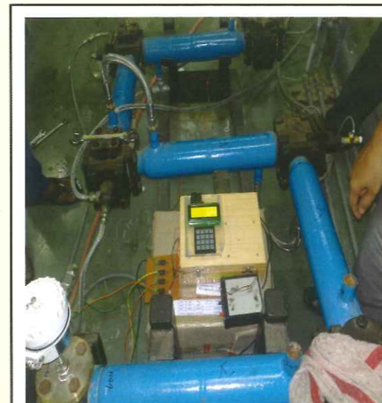
Wireless instrumentation for heat exchanger
